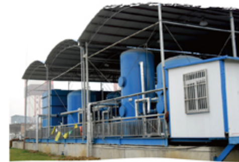
Water Purification Project of Anhui Development Mining
