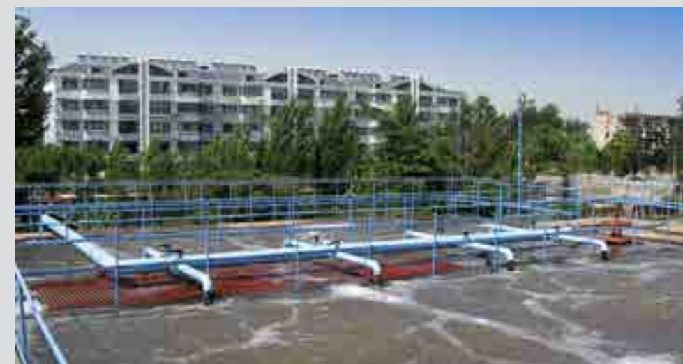
Sewage Treatment Station of Power Plant of Luzhong Mining Co., Ltd.
