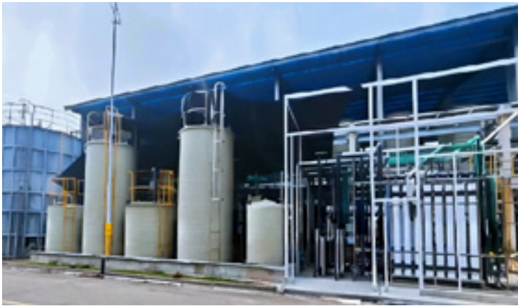
Wastewater Treatment Unit at the Tongguan Base
